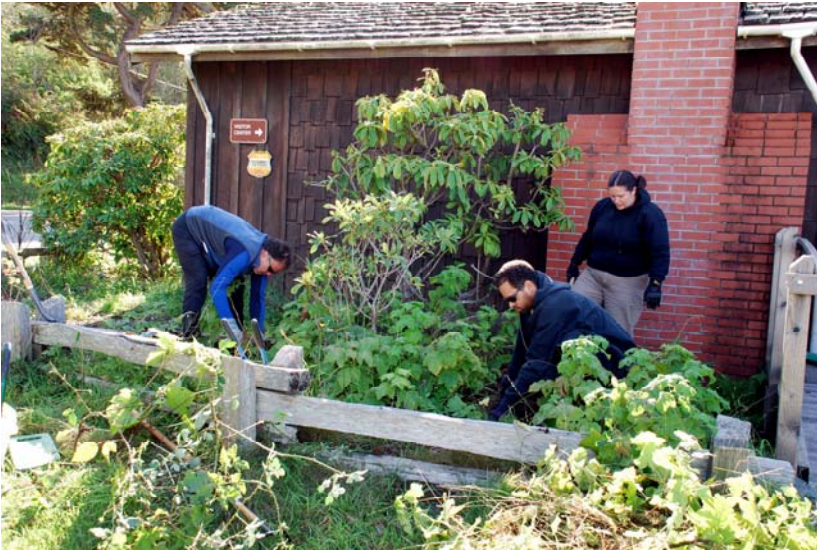
Stone Lagoon Visitor Center of Humboldt Lagoons State Park gets a native plant make-over. Prairie Johnston, Michael Moore and Vic Armijo clear blackberries, invasive grasses and other weeds before the second phase of native plant installation.
